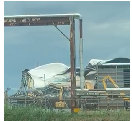
PHOTO: Improper covering of demolition activities is allowing radioactivity to move offsite.
